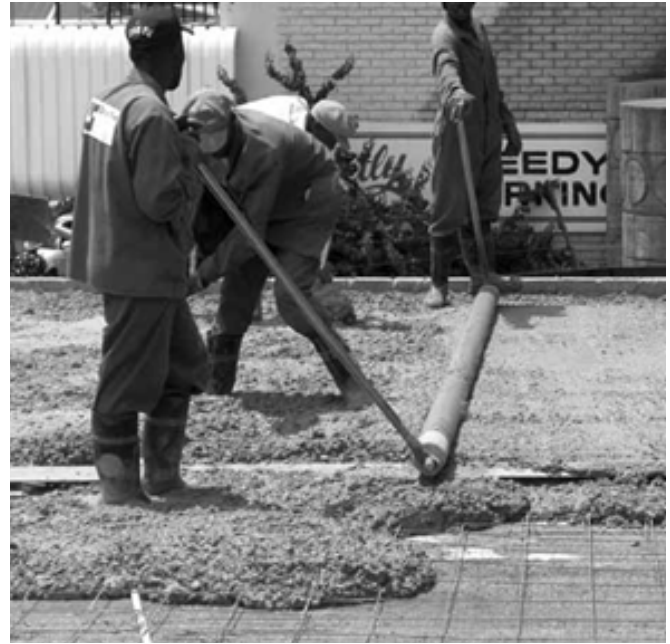
Leveling a concrete topping. Reinforcement and temporary screed battens in the foreground.
