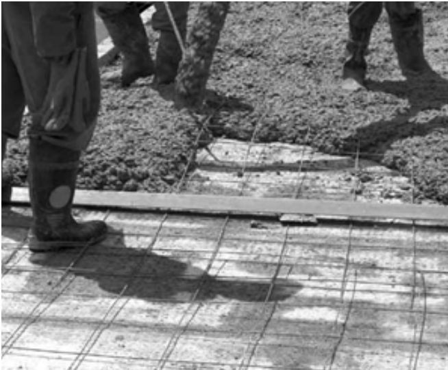
Pumping a concrete topping onto precast flooring. Reinforcement and screed battens in foreground.
